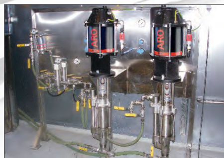
4-ball piston pumps, 4:1 ratio, installed on a paint formulation process
