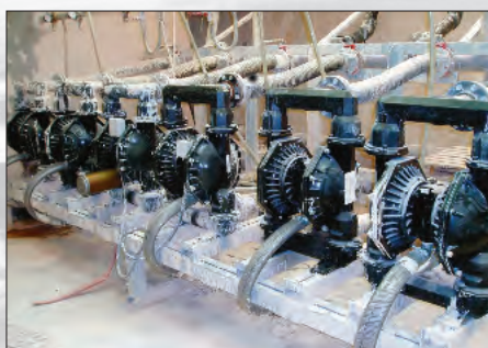
3" diaphragm pumps mounted on a skid to transfer clay in a ceramic manufacture
